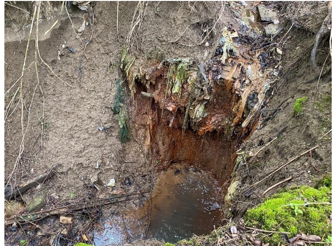
Lack of Maintenance
