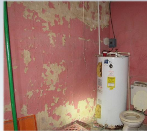
Deteriorating lead-based paint
