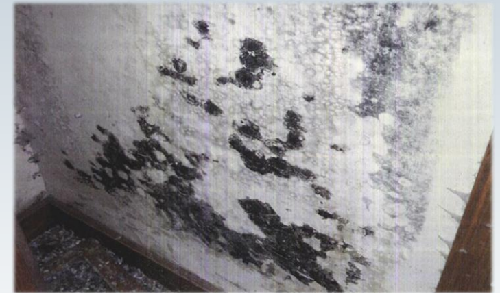
Mold growth on water-damaged wall
